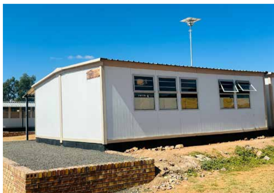
One of the school blocks constructed using containers, boasts 18 classrooms designed to accommodate 540 learners. Photo: Nothando Makhubela
