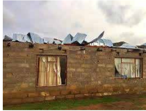
Roofs Destroyed, Families Left Exposed After Storm in Nkomazi. Photo: Supplied.
